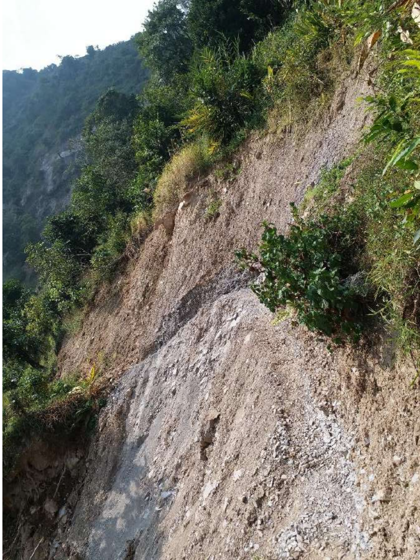
Photo:5 Landslide at Lamsarang
