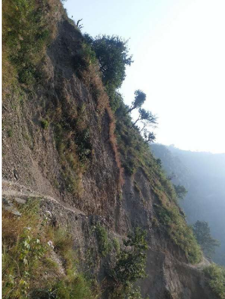
Photo:6 Landslide at Nayakhani
