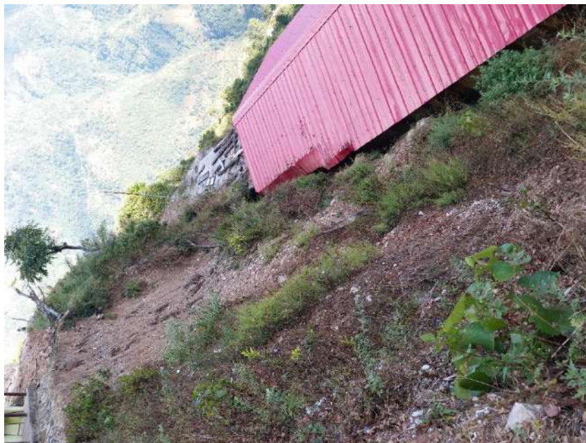
Photo:9 Landslide at Lung School
