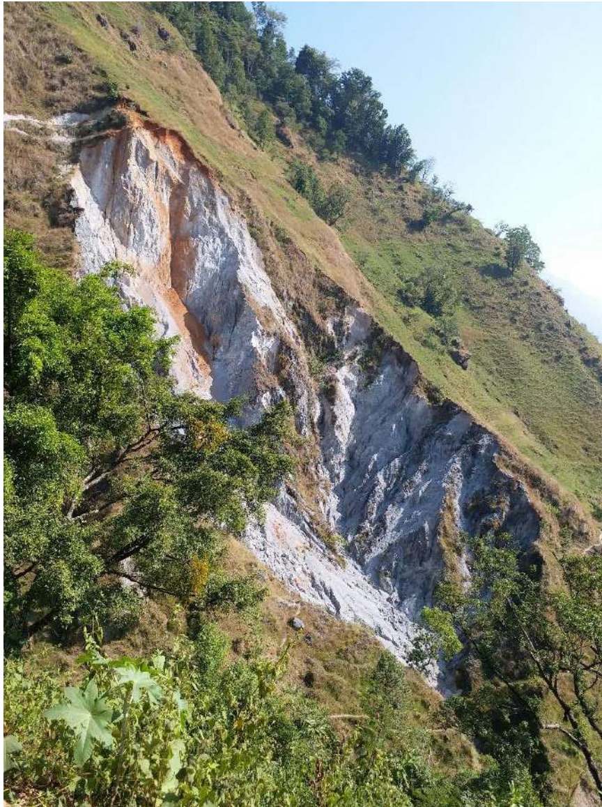
Photo:10 Landslide at Lower Korang
